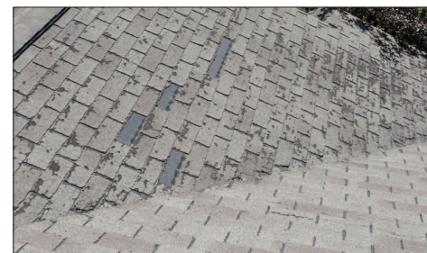
Lake Orion Roofing finds hail damage after inspecting the integrity of this homeowner’s roof. Damaged shingles are not as effective in protecting the home from further leaks.
