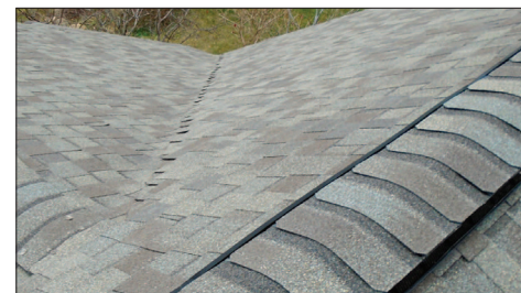
After working with Lake Orion Roofing the homeowners have new roof, guaranteed under the business’ workmanship. For a free assessment, call 248-393-0055. sure they are satisfied their first time around. And unlike the numerous door-to-door contractors who leave the state after a roof installation, we’re right here in your backyard.”
