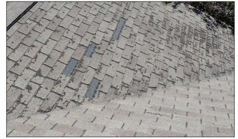
Lake Orion Roofing finds hail damage after inspecting the integrity of this homeowner’s roof. Damaged shingles are not as effective in protecting the home from further leaks.
